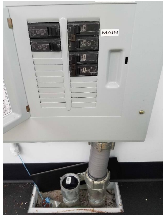
Existing electrical panel and stub up.
