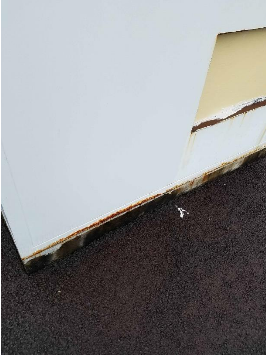
Surface corrosion at base of wall panel.
