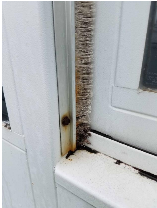
Surface corrosion at sliding window jamb.
