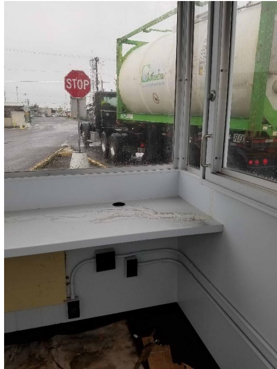
Existing countertop, window AC opening infill panel, electrical conduits and junction boxes.
