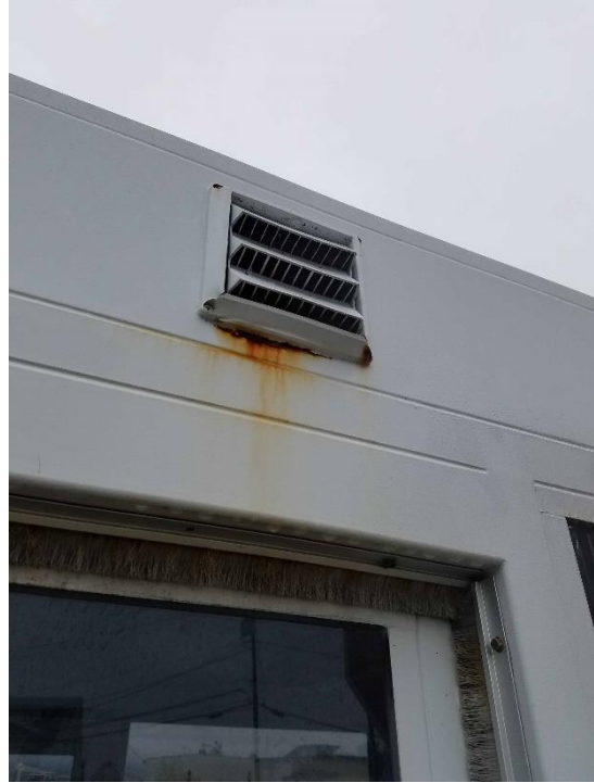
Surface corrosion at attic vent.
