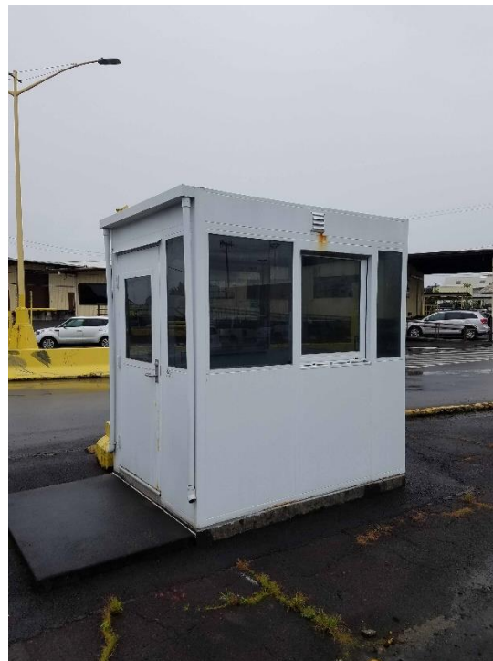
Side and rear view of existing guard shack. Note concrete base, landing, and downspouts.
