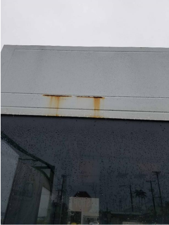
Surface corrosion at wall panel.
