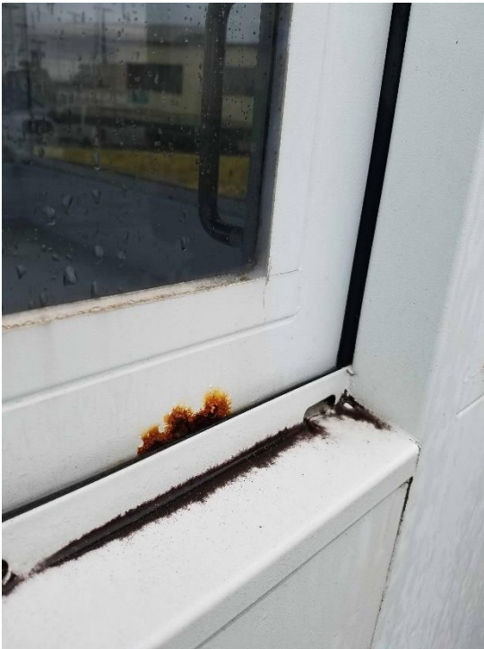
Surface corrosion at sliding window.
