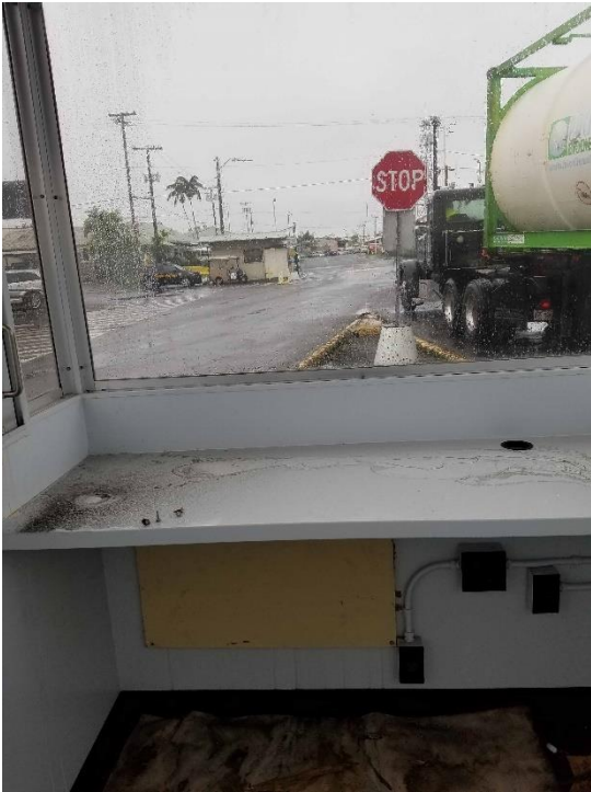
Existing countertop, window AC opening infill panel, electrical conduits and junction boxes.
